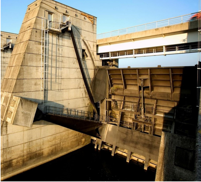
Figure 3. Radial hydraulic gate. Source: CNR.
