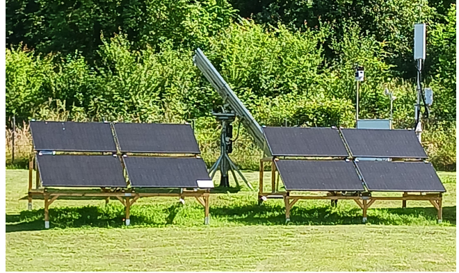
Figure 1. Photograph of the FHC twin-plant PV installation used for data collection.
