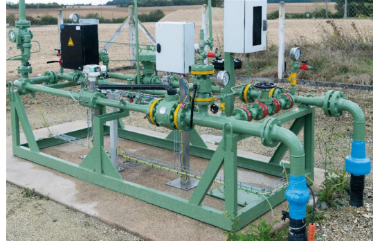
Figure 1. Gas pressure reduction and delivery station
