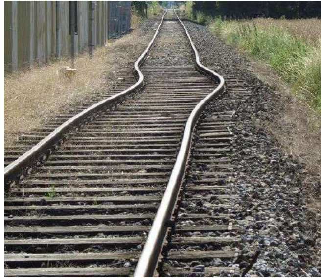
Figure 4. Unacceptable condition of the track
