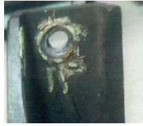
Figure 6. The oval form detected in one of four holes points to bolt loosening
