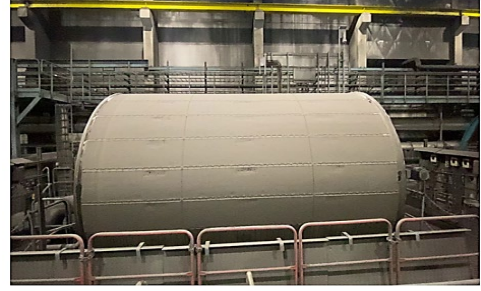
Figure 4. RVDF during normal operation.
