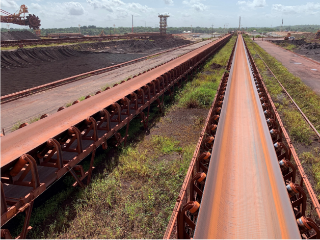
Figure 1. Belt conveyors in iron ore yard (Carvalho, 2022).
