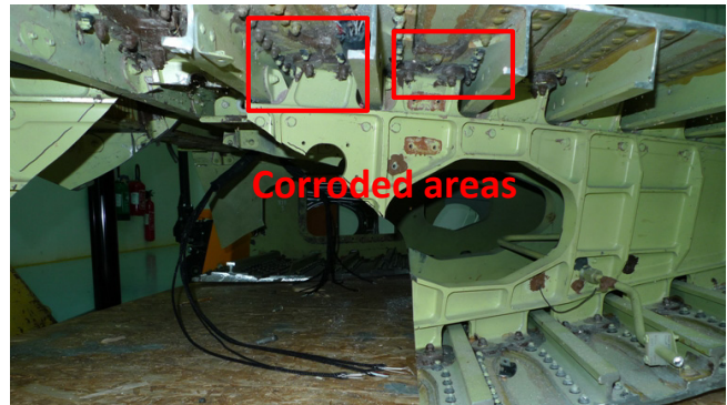
Figure 14. A320 wingbox with corrosion flaw inside the wing. (Acknowledgments to Airbus and EADS-IW)
