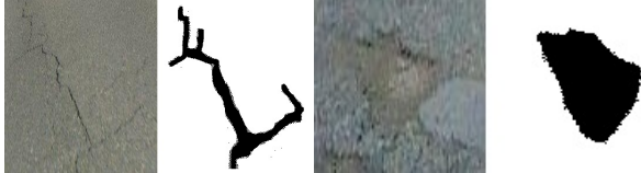
Figure 3. Road damages and their segmentation masks. From the left, the first and the second images show a linear crack and the segmentation mask, respectively. The third and the fourth show a pothole and the segmentation mask.
