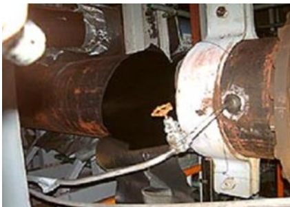
Figure 1. Pipe wall-thinning accident of Mihama plant.
