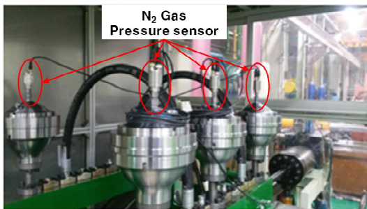
(a) N 2 Gas pressure sensor
