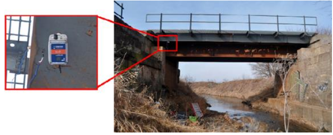
Figure 15. Testing a wireless sensor network on a railway bridge (Fu et al. 2018)
