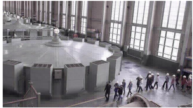
Figure 9. Hydro-Québec generating unit
