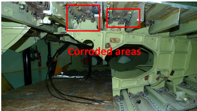
Figure 14. A320 wingbox with corrosion flaw inside the wing. (Acknowledgments to Airbus and EADS-IW)
