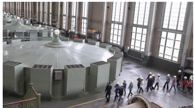
Figure 8. Hydro-Québec generating unit photography. A group of experts have been involved to identify possible failure mechanisms for the stator of hydrogenerators based on a literature review and their own experience. Three failure modes have been identified for the stator, as presented in Figure 9, and over than one hundred failure mechanisms have been identified as possibly occurring in the stator of hydrogenerators. Over seventy different physical states have been defined. The causal graph representing all failure mechanisms of the stator is presented in the figure 9 bellows.
