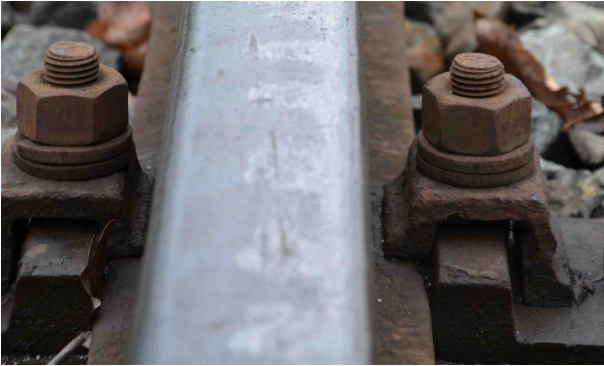
Figure 1. Corrugated rails reduce the driving comfort in terms of vibration and noise while increasing the overall wear due to harsher track - train interactions.
