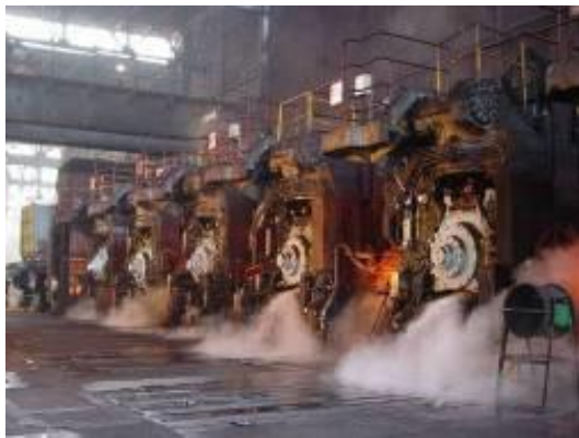
Figure 2. Hot Strip Mill at Florange
