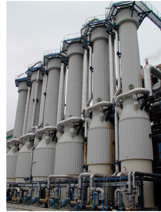
Figure 1. Five evaporation units for the evaporation section in a beet sugar factory in Spain.
