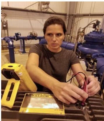
Figure 16: Measuring a thermal age tag attached to an electrical motor at a municipal water facility. The tag projects remaining winding insulation thermal life.
