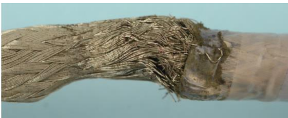
Figure 14. Actual wire damage after teardown of H1
