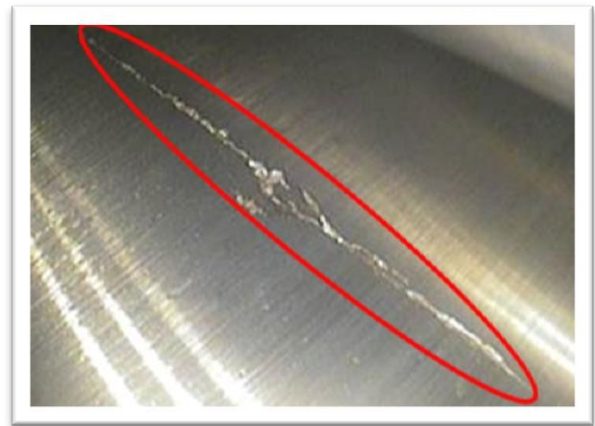
Figure 9. Bore scope inspection of the inner race
