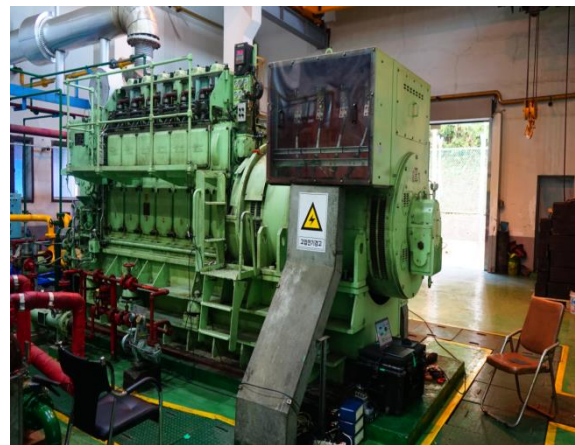
Fig. 1 Overview for diesel generator at the diesel power plant of a small island
