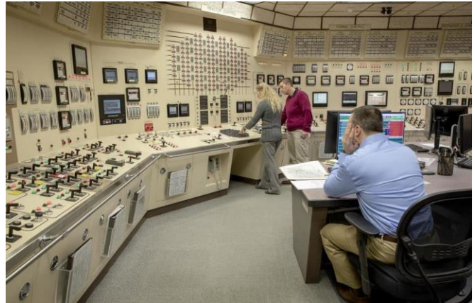
Figure 3: Entergy's Chiltonville Training Center is an identical twin mock-up of the control room at the Pilgrim nuclear power plant. (R. Lubbock, 2019)
